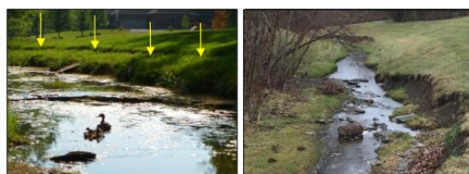
Stream erosion may start as a tension crack along the bank (left) that eventually leads to bank collapse and widening (right)
