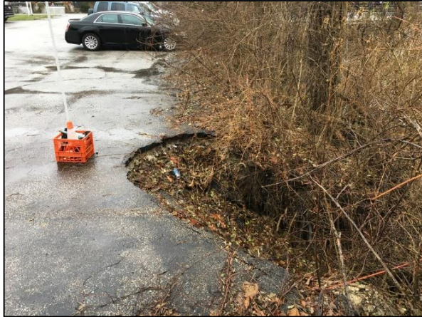
Stream erosion undermining parking lot → public safety risk
