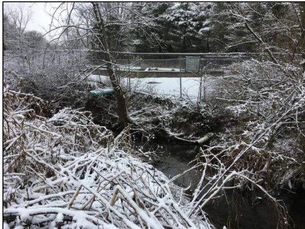
Exposed pipes in bank show extents of bank erosion near Wastewater Facility
