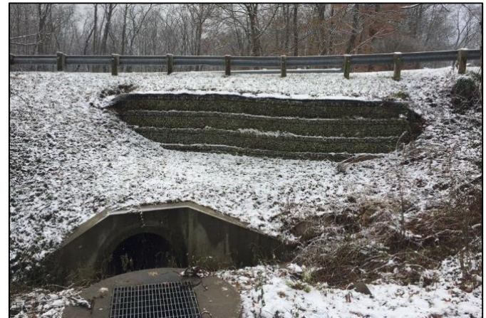
Slumping gabions next to road
