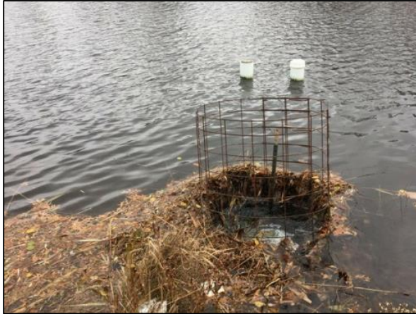
Existing outlet structure that could potentially be optimized to reduce downstream erosion.
