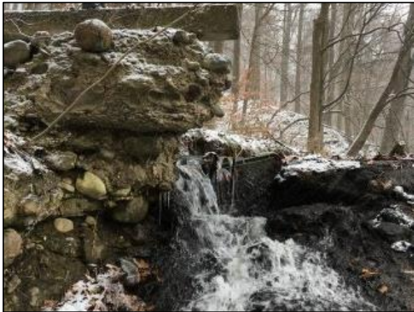
Dam is patched with a piece of plywood & chain-link fence
