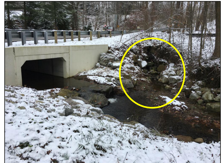
Outlet would benefit from additional armoring and stabilization
