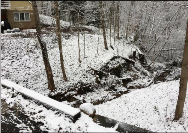
Eroded ravine downstream of driveway.
