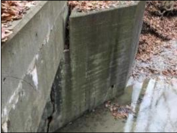
Cracked bridge abutment
